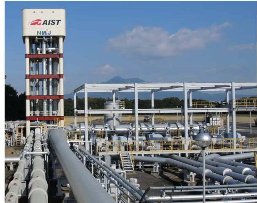
Water flow facility
